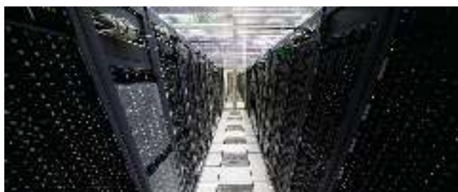
Figure 13.15: Data storage facility.
